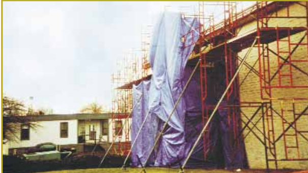
Foreground: damaged credit union exterior. Background: temporary credit union office keeps customers happy.
