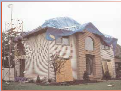
Before and after photos of the exterior reveal, at left, heavy fire damage to the fireplace and roof "made right again" by Allen Keith Construction, at right.
