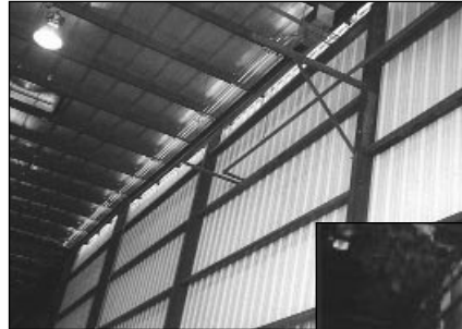
Interior view of damaged wall and roof (below), “made right again” (at left).
