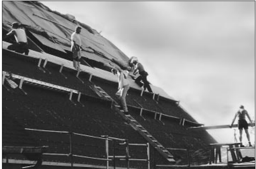
Allen Keith construction crew replaces north side of sanctuary roof—making it right again, one board at a time.
