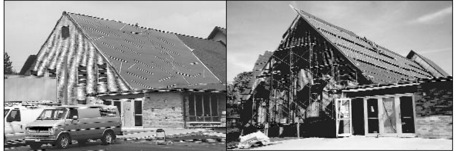
Over 7,000 square feet of tarpaulins provide temporary protection (left). At right, all roof sheathing has been replaced, with installation of new shingles nearly complete.
