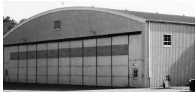
The roof of this Air Camis building was completely replaced by Allen Keith Construction.
