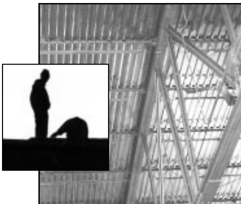
New roof applied by Allen Keith Construction. Inset: Workers silhouetted against skies over Canton-Akron Airport.
